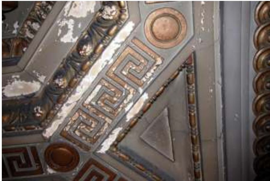
A typical water-damaged area on the southwest side of the lower entry stairway ceiling.
