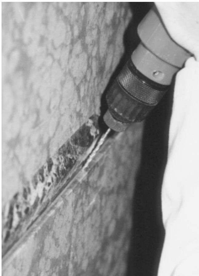
Figure 9. A 0.08-cm ( 1/32 -in.) hole drilled at 45^\circ to accept the tail of the mechanical fastener.
